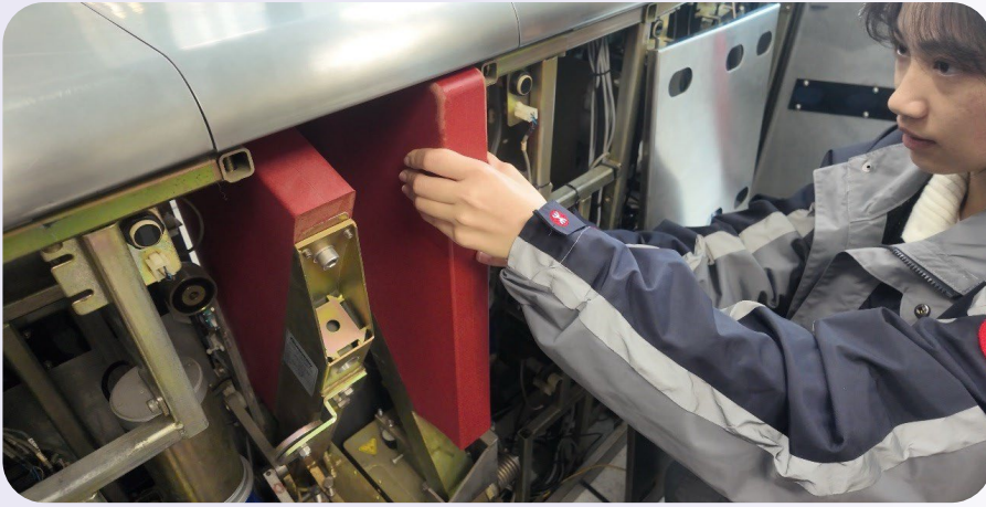
大客流控制板現場安裝與調試 On-site installation and commissioning of the high-passenger-flow control panel
